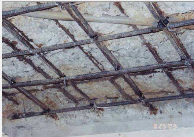
2.鋼筋剪薄量過多處鋼筋綁紮
